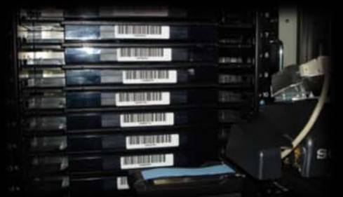
Flexicart Internal view Elevator & Barcode reader
